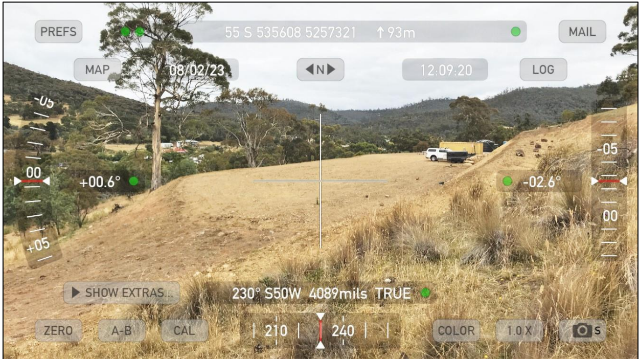
Photo 13 – Cut-and-fill at the eastern end of the development site, with proposed house site at centre
