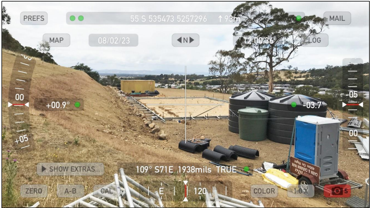
Photo 9 – Cut-and-fill at the western end of the development site, with proposed shed site at centre
