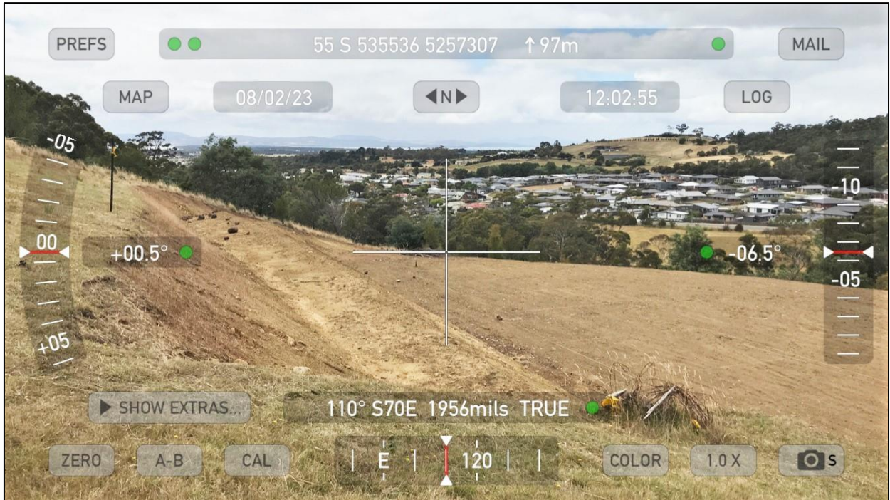
Photo 11 – Cut-and-fill at the eastern end of the development site, with proposed house site at right
